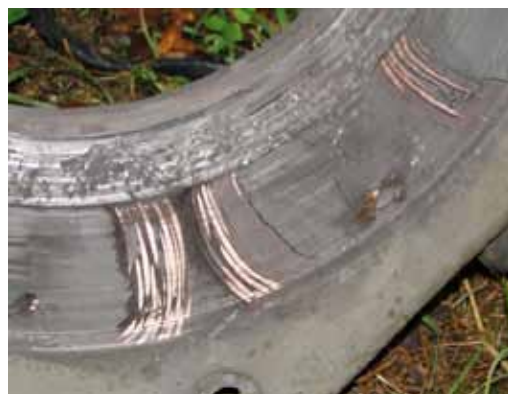
Fig. 34: Stator that needs to be changed
