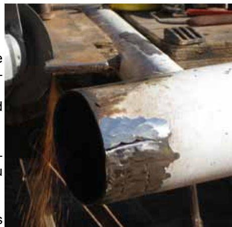
Fig. 44: Crack in the tail pipe
