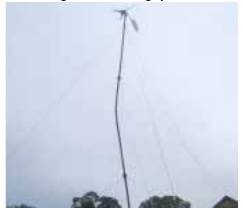
Fig. 68: Tower too tight
