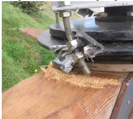
Fig. 67: Threaded rod too long
