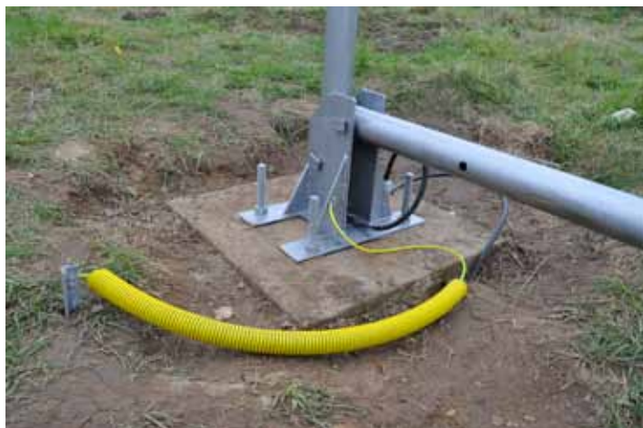
Fig. 2: Ground connection of the tower and electronics
